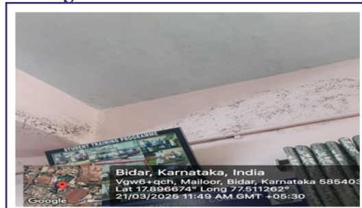
Fig. 1: Moisture occurred beam
