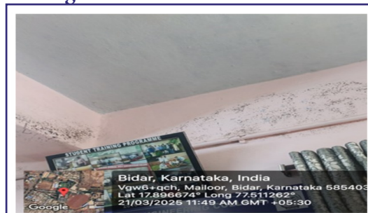
Fig. 1: Moisture occurred beam
